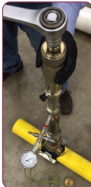
Camera Fitting Set-up
